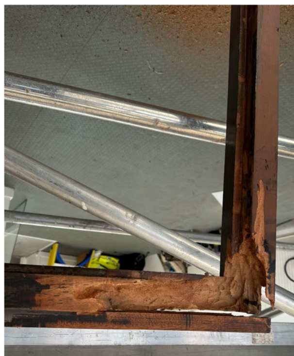
Window removed from frame and rot discovered
