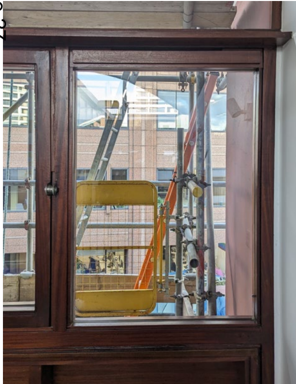
Internal view of trickle vent
